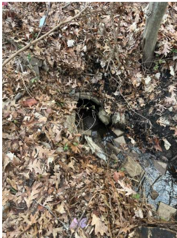
12" Diameter Outfall to the West of the Development Area
