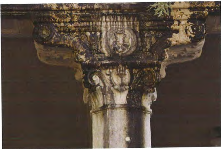
Details to be restored Image taken by HLW
