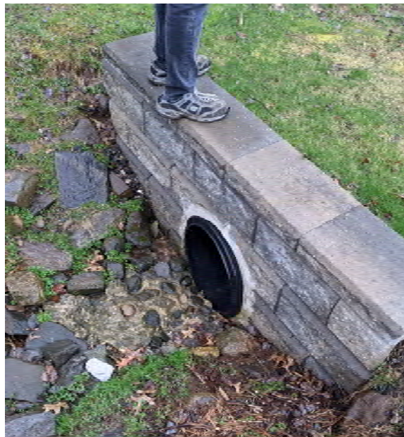
Figure 4. Origin of 24" HDPE Pipe (inlet), located behind 14 Dean Road.
